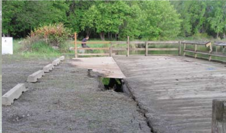
Damaged Gilbert River ADA Fishing Pier
